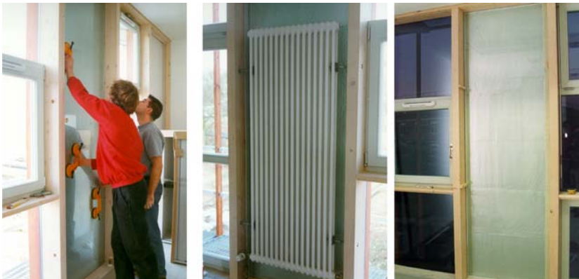
Fig. 14. In 1998 first installation of VIPs in a building at the test façade of ZAE Bayern. For testing purposes VIPs were integrated into the spacing of a jamb-crossbar construction.
