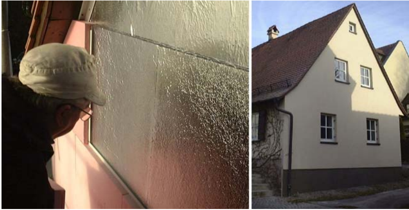
Fig. 15. Gable façade of an old building under protection during the installation (left) and after renovation was finished (right). The shiny VIPs are in a rail system. The pale pink polystyrene boards have just been mounted.
