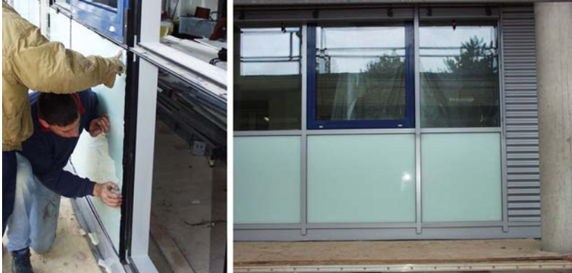
Fig. 17. Jamb-crossbar construction made of aluminum: vacuum-insulated facade-elements during the installation (left) and outside view of the façade (right).
